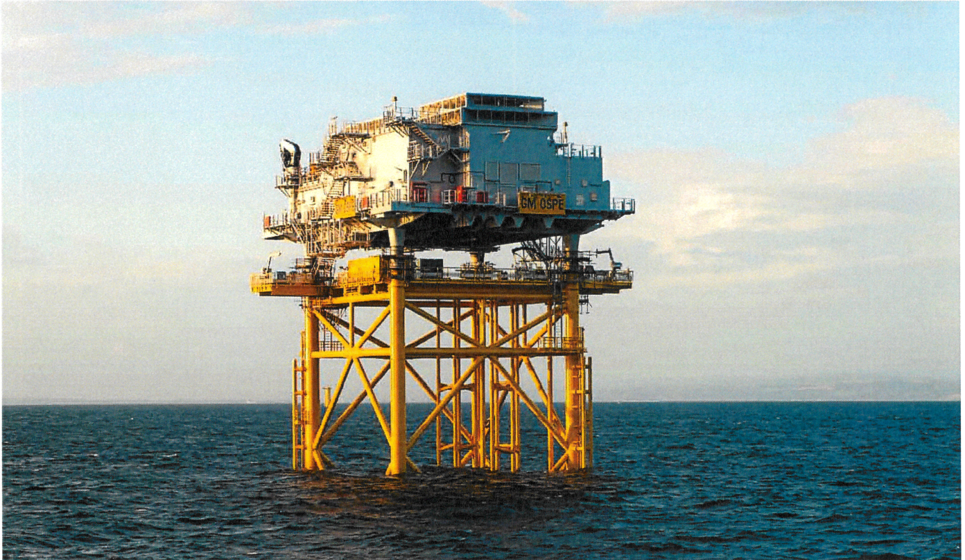
One of the two offshore substations installed in Liverpool Bay for Gwynt y Môr
